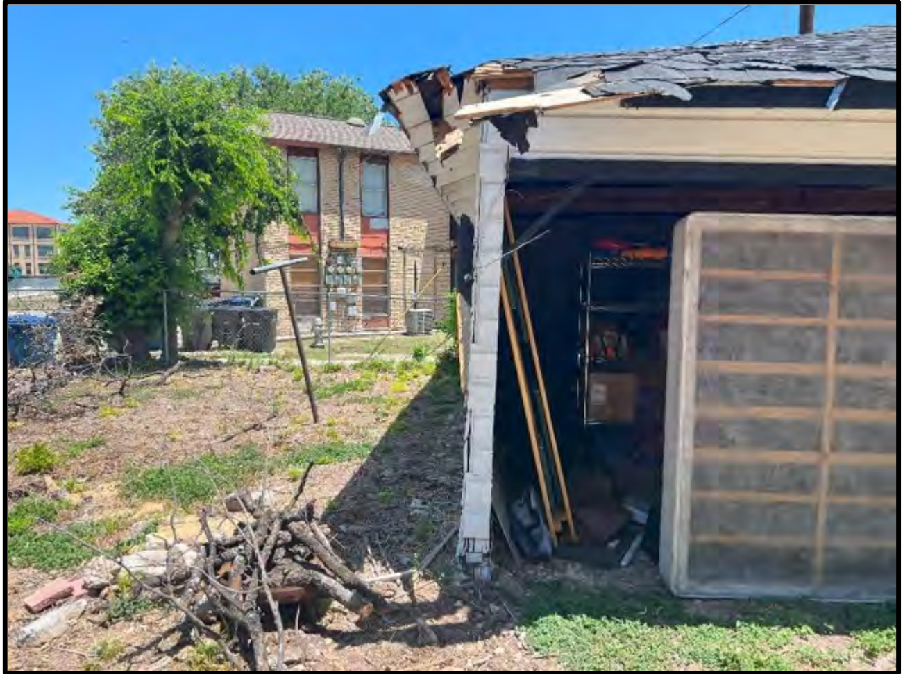
View of the impact area at the southwest corner of the detached garage building.
