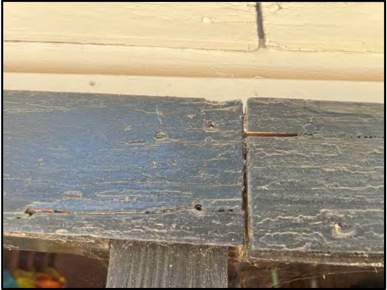
View of split cracks on the trims at the front (south) of the detached garage building.
