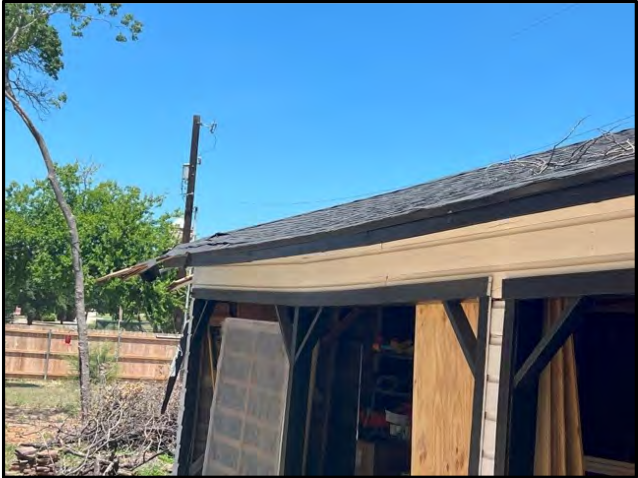
View of a deflection deformation of the opening header at the front (south) of the detached garage building.
