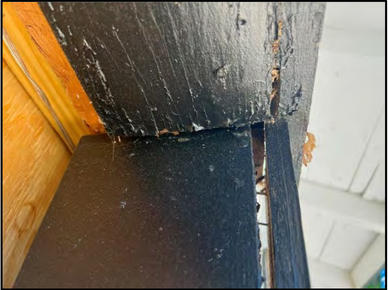
View of displaced frame and trim at the front (south) of the detached garage building.
