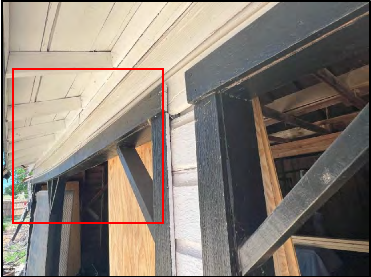
View of a deflection deformation of the opening header at the front (south) of the detached garage building. Note partially detached trim boards.
