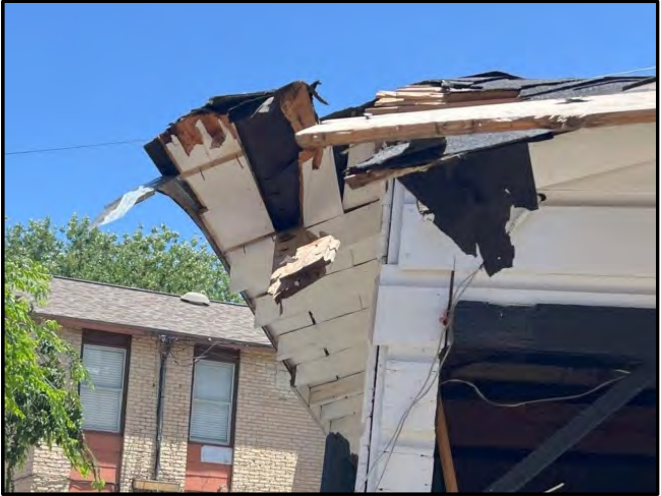
Close-up view of the impact area at the southwest corner of the detached garage building.
