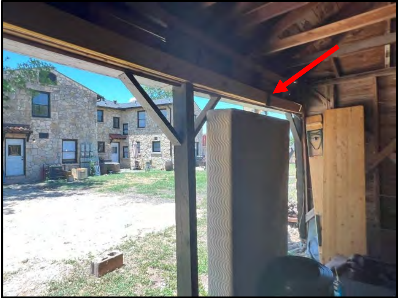
View of a deflection deformation of the opening header at the front (south) of the detached garage building.
