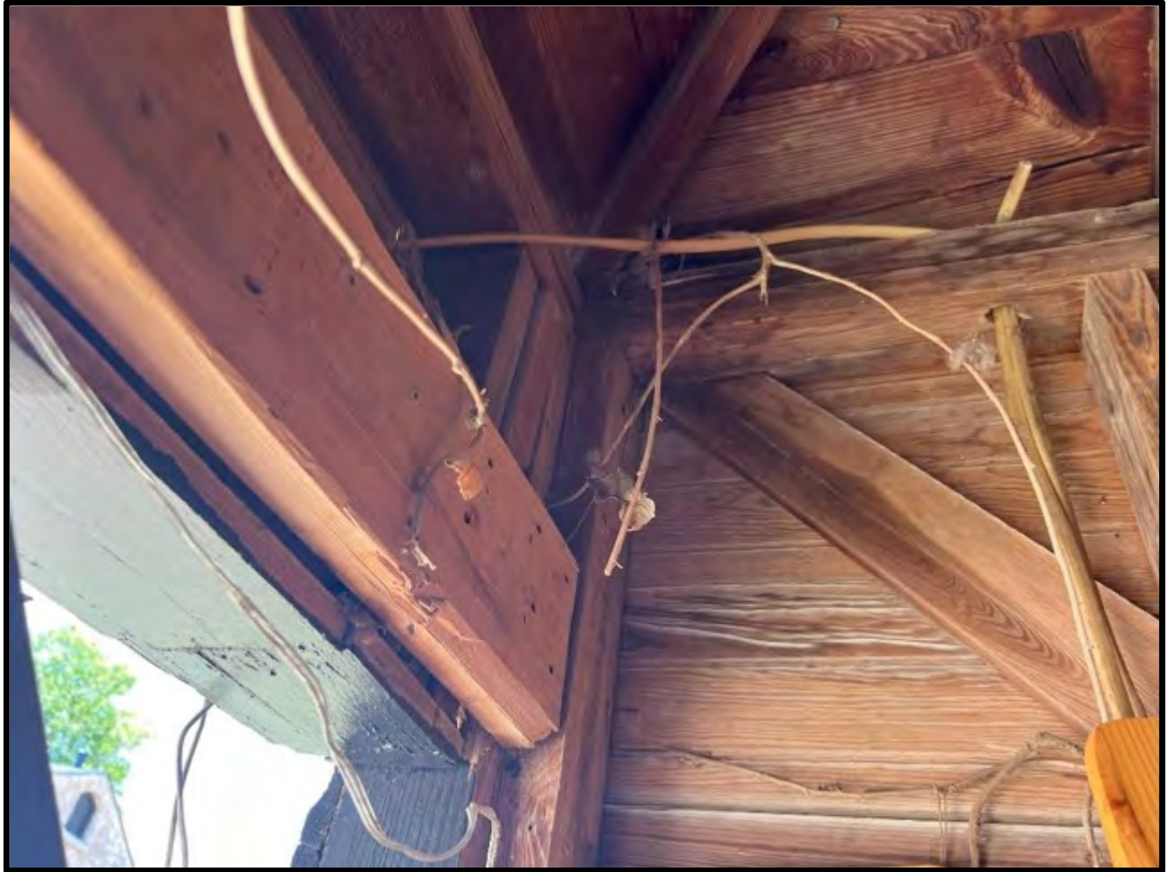
View of a displaced header (beam) from a column post at the southwest corner of the detached garage building.
