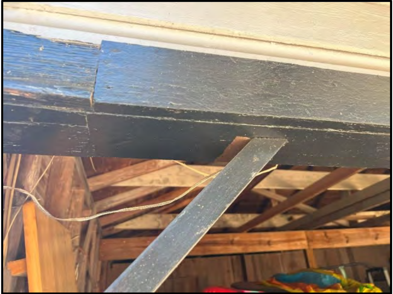
View of displaced bracing member at the front (south) of the detached garage building.
