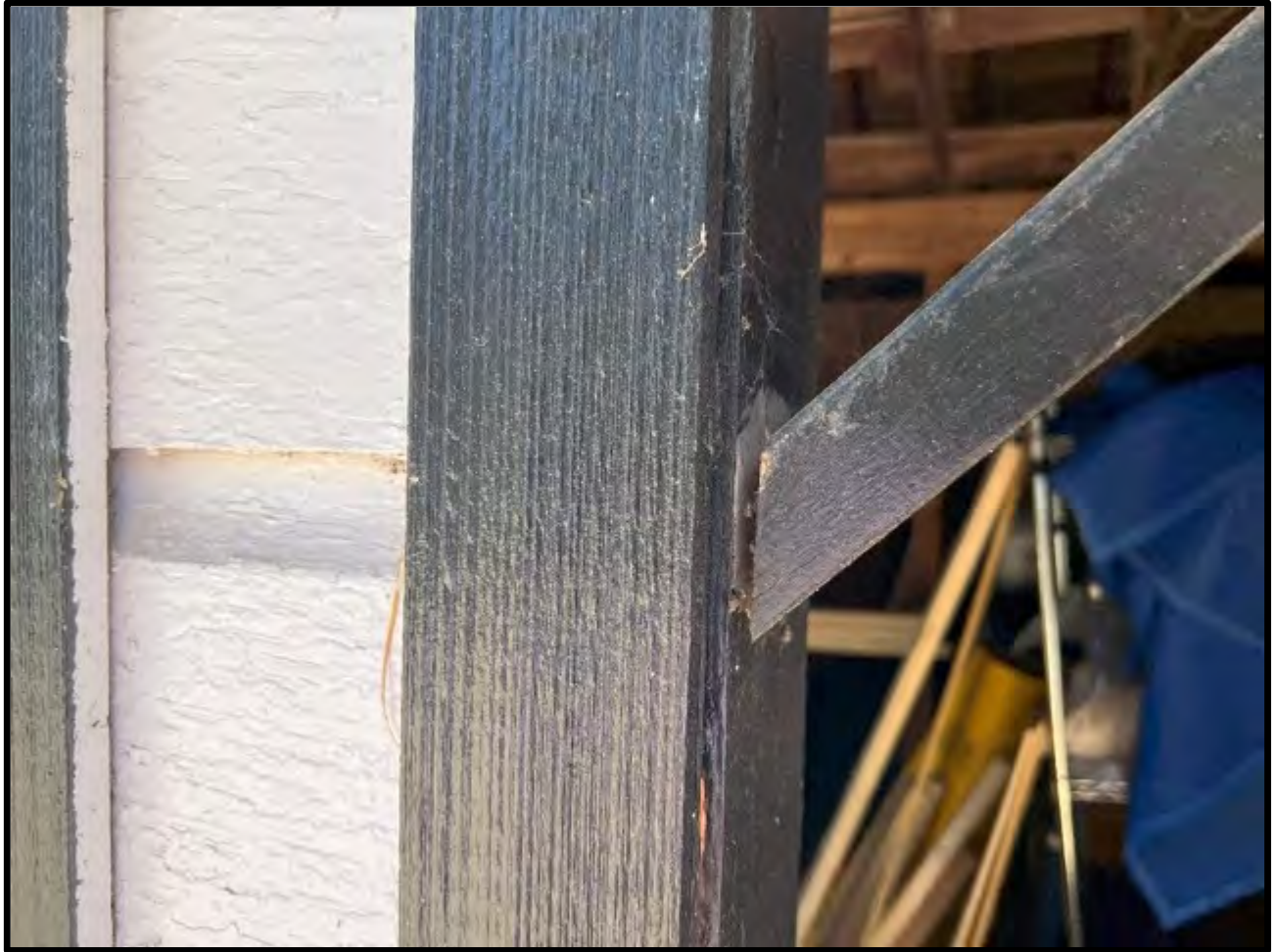
View of displaced bracing member at the front (south) of the detached garage building.
