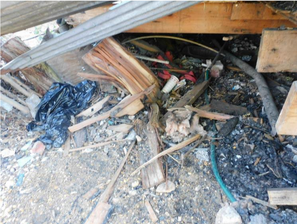
Photo 11, Crawlspace, damaged foundation pier.
