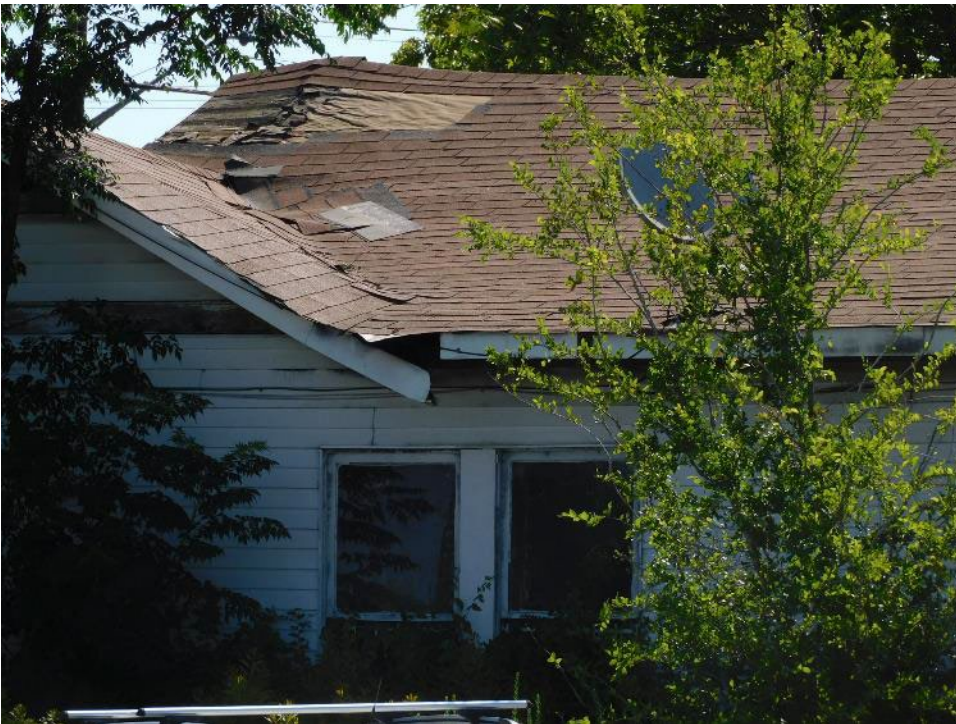
Photo 12, Exterior, damaged roof, east elevation.
