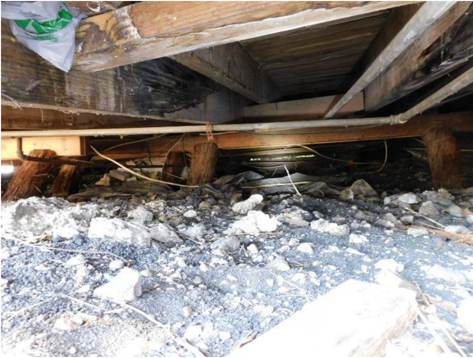
Photo 9, Crawlspace, toppled foundation piers.
