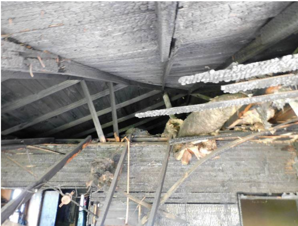
Photo 8, Attic, damaged roof framing.
