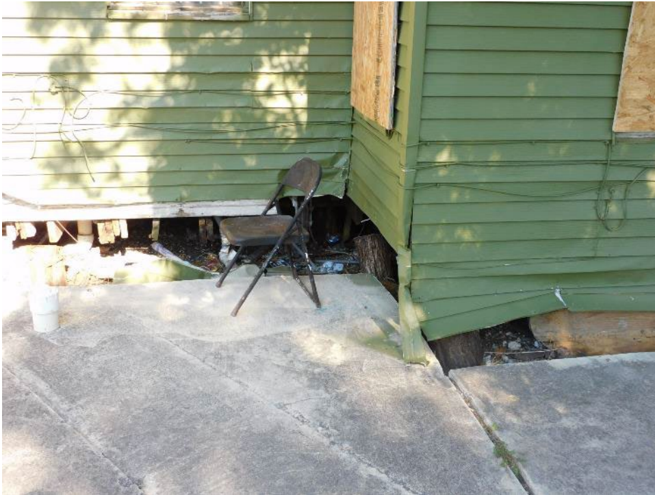
Photo 5, Exterior, damage to skirting and cladding, east elevation.
