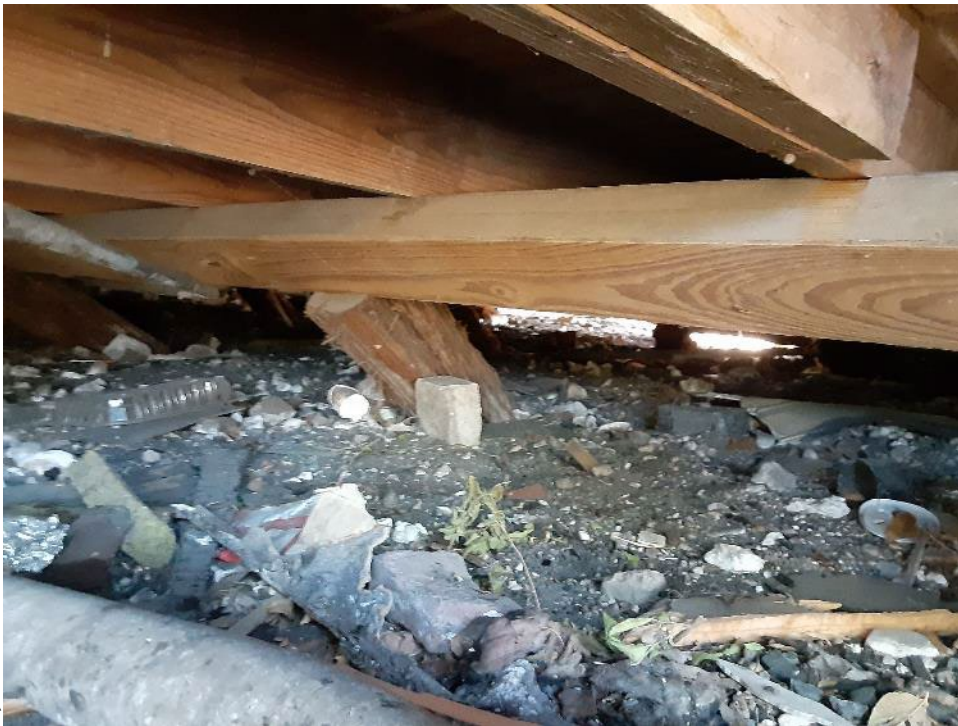
Photo 10, Crawlspace, toppled piers and rolled wood beam.
