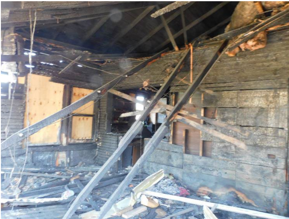
Photo 6, Interior, damage to framing and walls.
