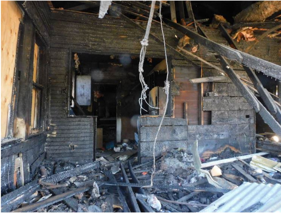
Photo 7, Interior, damage to walls and framing.
