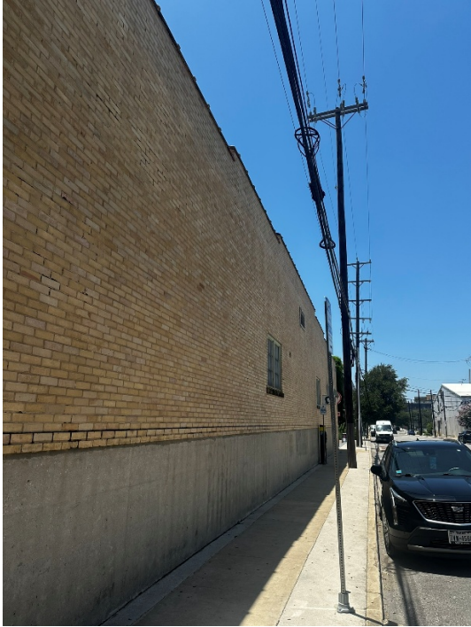
Figure 2. North Side of Garage Building shows slab is 3-4 feet above sidewalk level, complicating efforts to connect sidewalk to FFE. Sidewalk is 4'9" wide on the level portion. The added sidewalk on the right is greater than a 2% cross-slope and is not code compliant.
