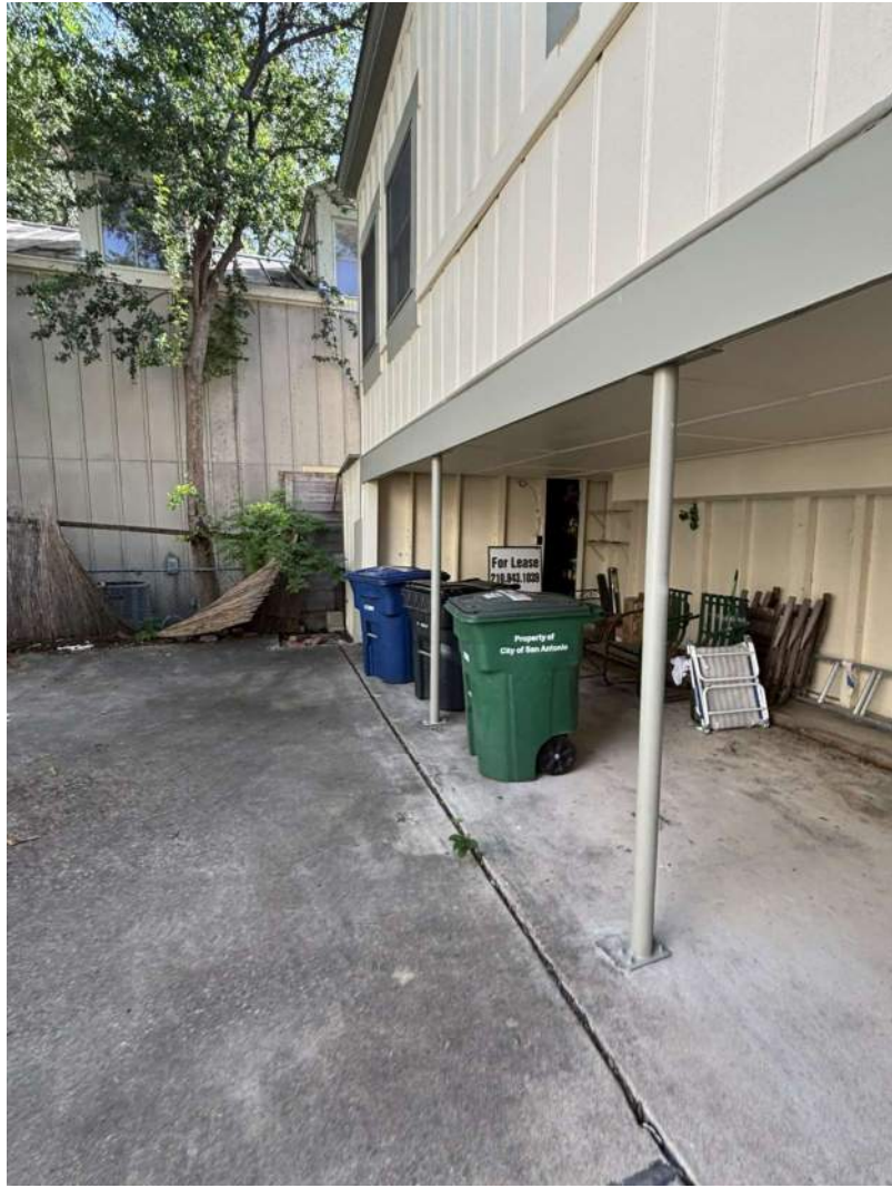
LOW CLEARANCE AT EXISTING LOWER LEVEL OF CARRIAGE HOUSE.
