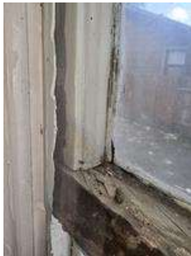
Location: Bedroom 2 Notes: -Damage to frame
