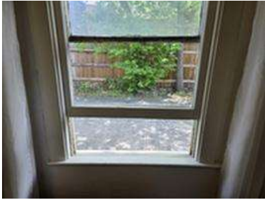
Location: Bedroom 2 Notes: Rotting frame, missing apron
