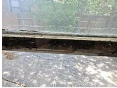
Location: Bedroom 2 Notes: water damage, wood rot
