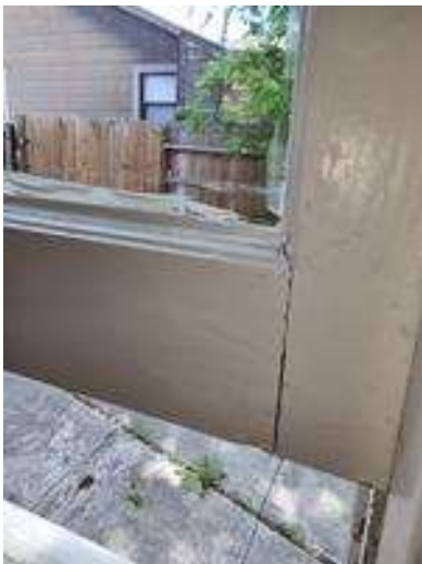
Location: Bedroom 2 Notes: -Cracked frame -Water damage
